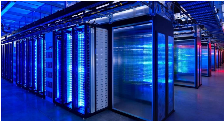
Figure 1: Hyperscale data centres will more than 100 racks housing hundreds of thousands of servers
